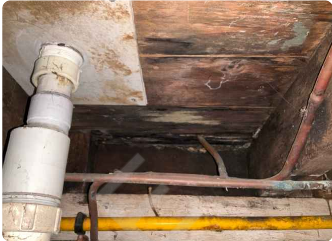
Showing example of damage
