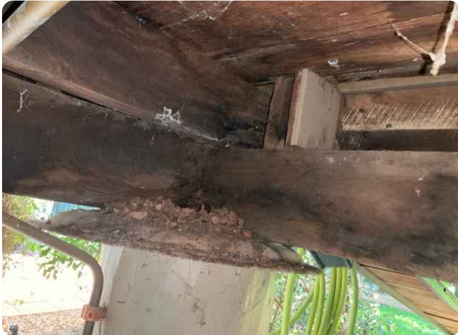
Showing example of damage
